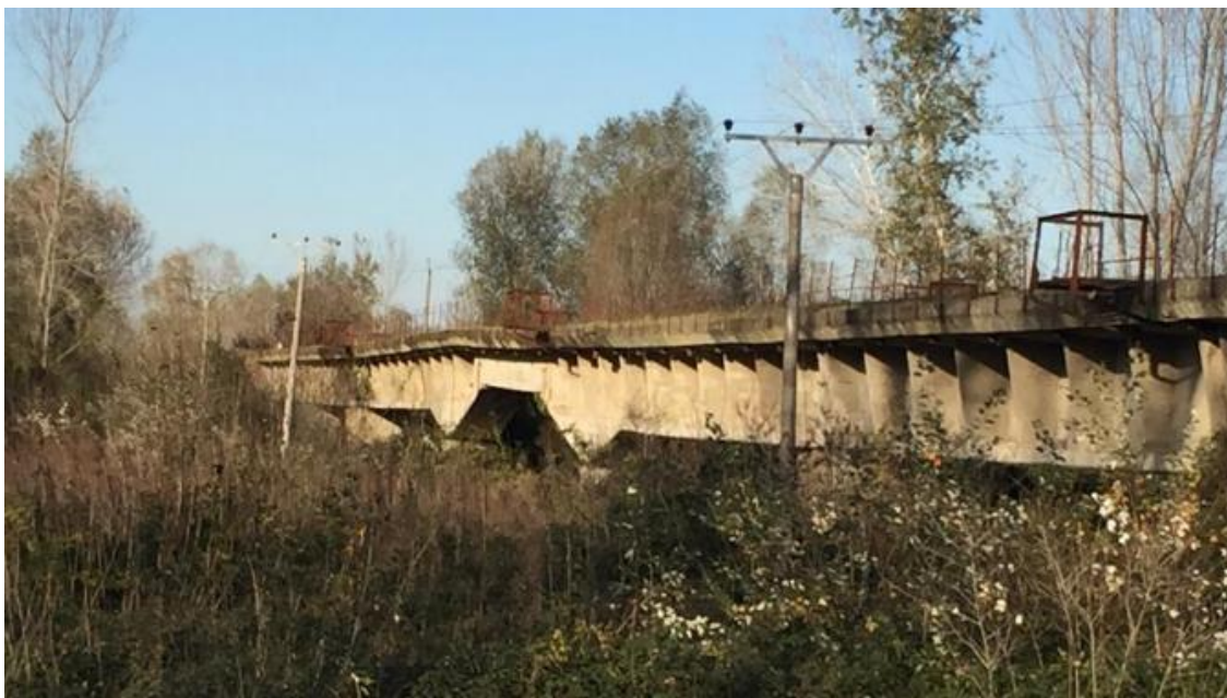
Figure 5.116_Linje elektrike e tensionit te ulet prane ures se Ishmit(km 35+100)
