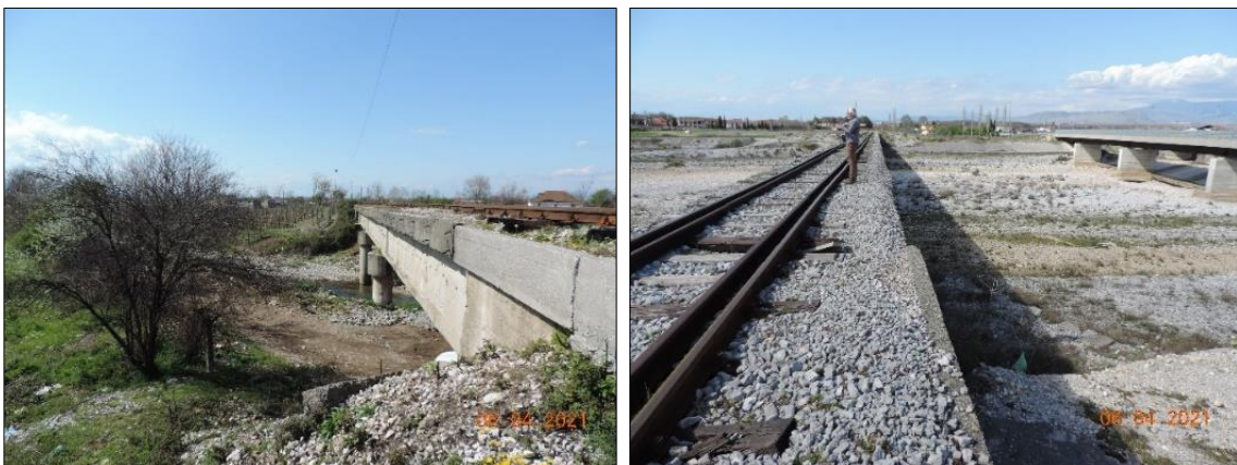
Figure 5.95_Majtas: Ura mbi kanalin e Vrakes; Djathats: Ura mbi perroin e Rrjollit
